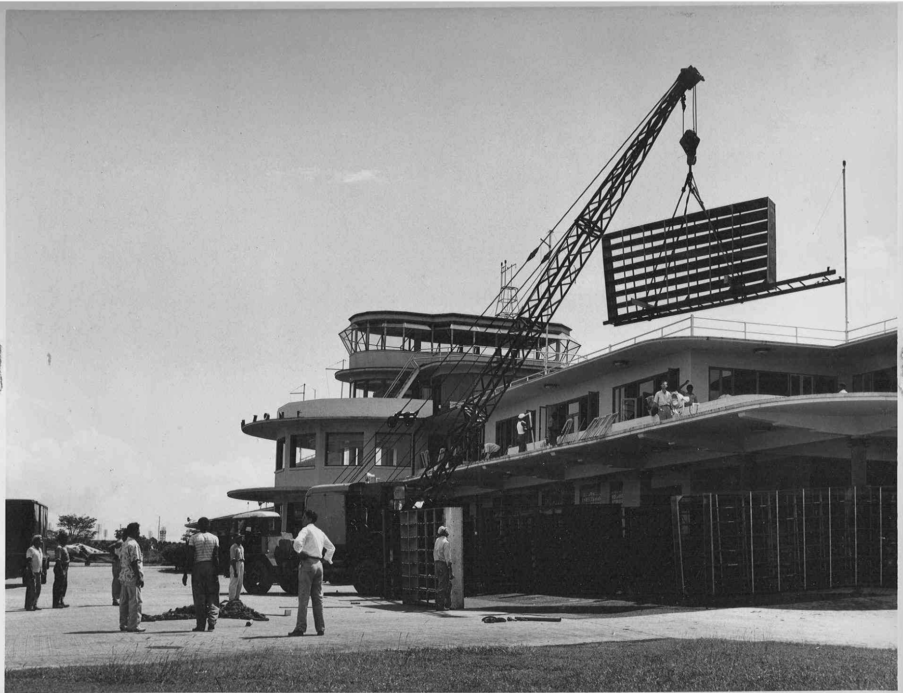
13-M-7(3) Panama Canal Library Equipment being moved into new offices at C. Z. Air Terminal, Oct. 26, 1949
